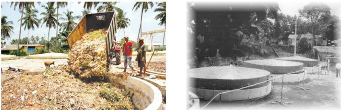
Figure 3: A batch type digester established in Dikovita- Sri Lanka
